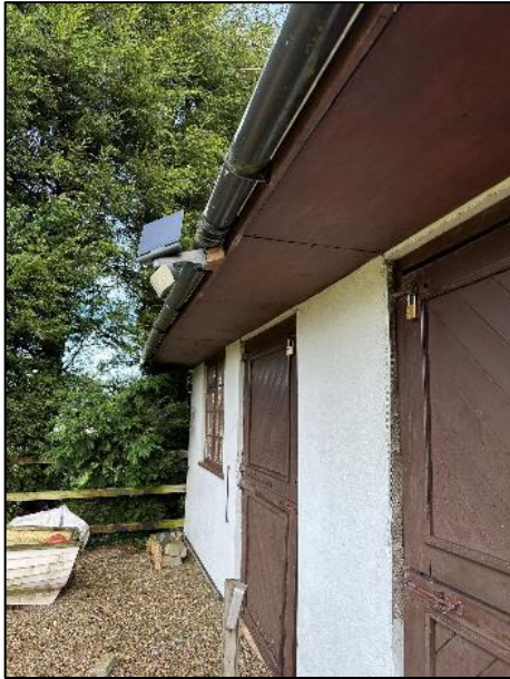
Photograph 44: No gaps between wood boards and main structure.
