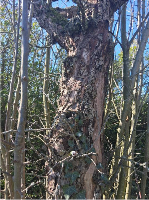
Photo 9: Deadwood observed on tree T1.
