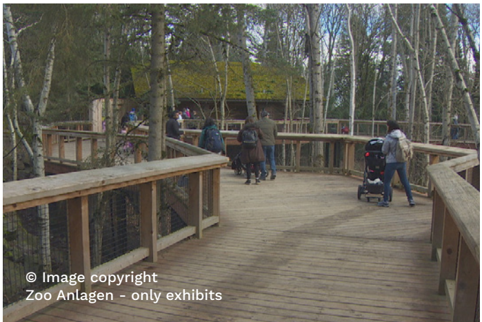
Standard timber post and mesh gaurding for boardwalks
