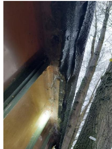
Plate 4.12: No gaps along the eaves
