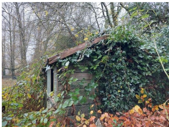
Plate 4.18: Hut with rotting timbers on roof
