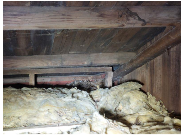
Plate 4.10: Bird nest in north-east corner
