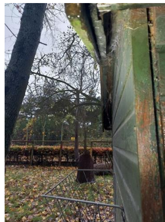
Plate 4.15: No gaps along the eaves
