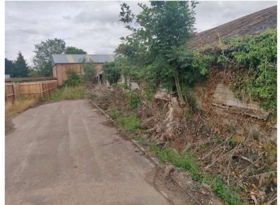
Photo No.18: Facing east showing the rear (southern) face of the linear barn, dilapidated state and further PACM
