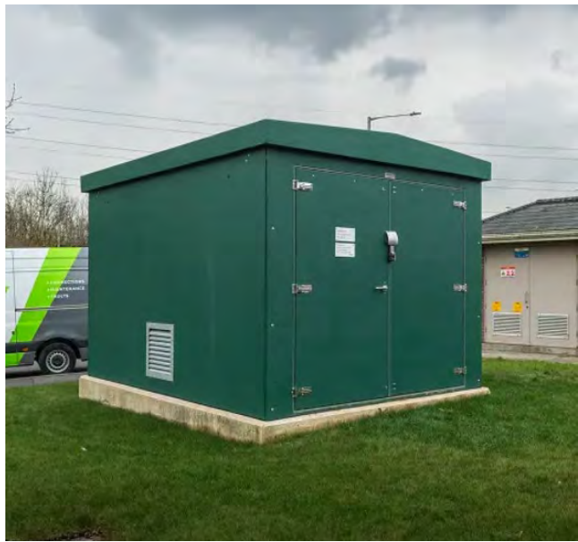
Typical Sub-Station enclosure
