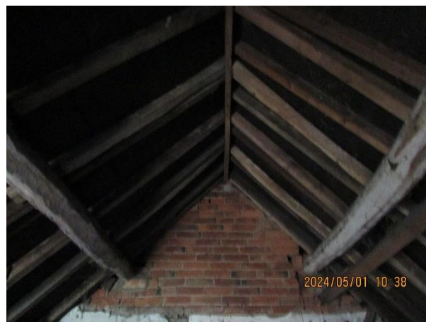
Exposed ridge and gaps in internal wall
