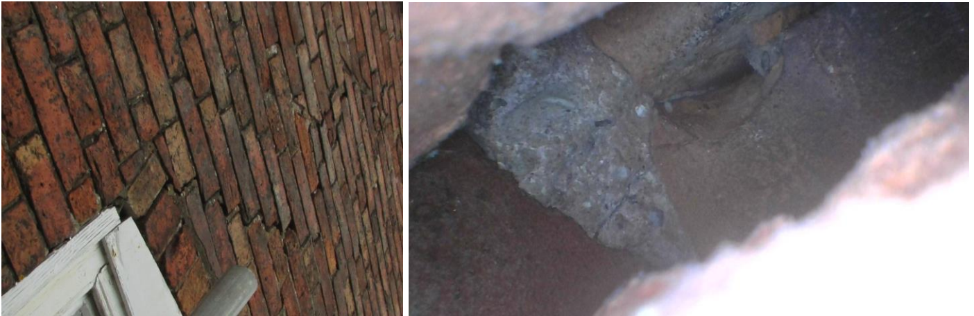
Crevice within southern gable wall
