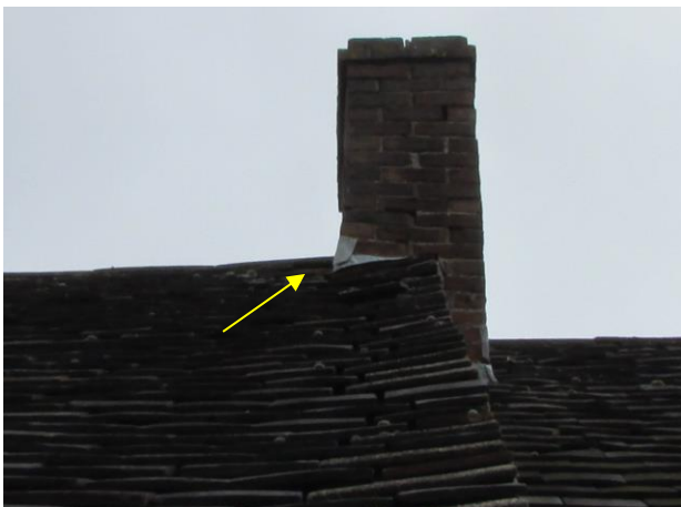
Damaged ridge tile
