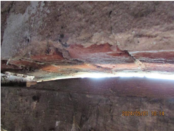
Gap above window
