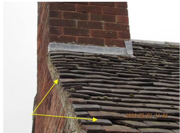
Damaged and lifted slope tiles
