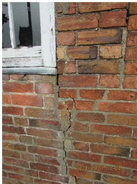
Crevice within southern gable wall
