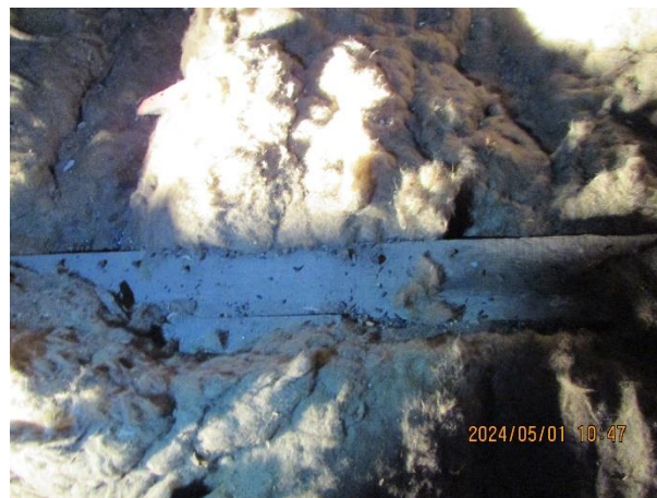
Bat dropping identified amongst mouse droppings
