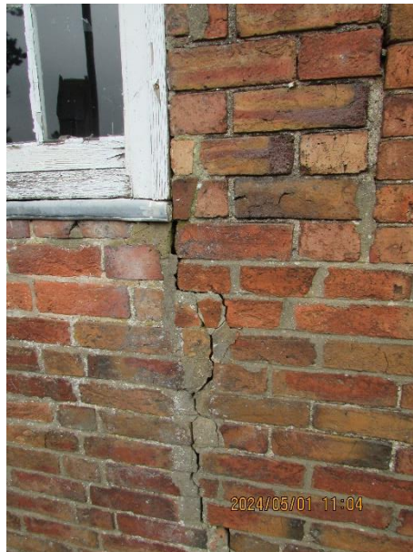
Crevice within southern gable wall
