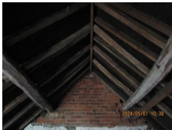
Exposed ridge and gaps in internal wall
