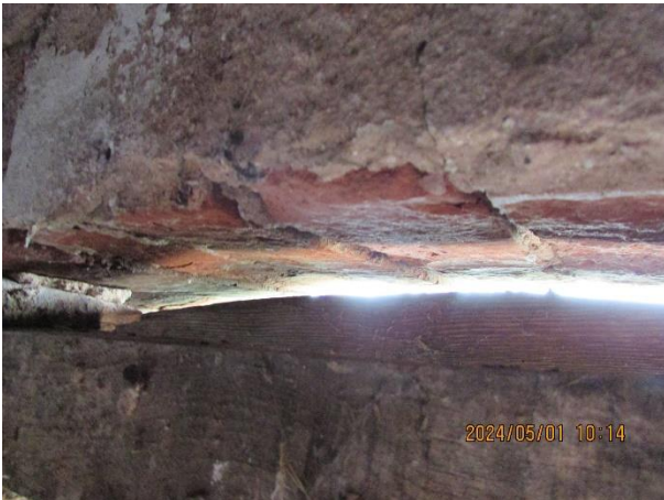
Gap above window
