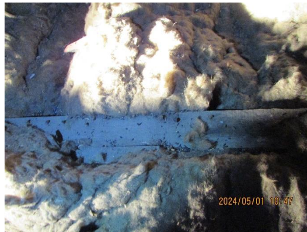
Bat dropping identified amongst mouse droppings
