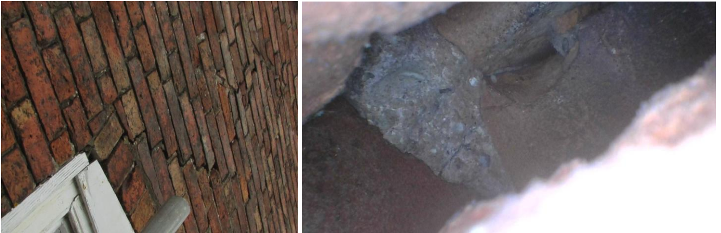
Crevice within southern gable wall
