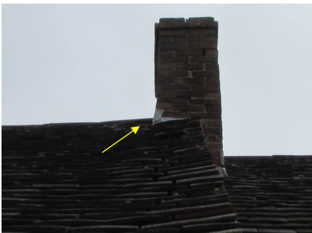
Damaged ridge tile
