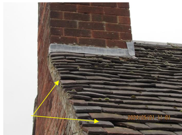
Damaged and lifted slope tiles
