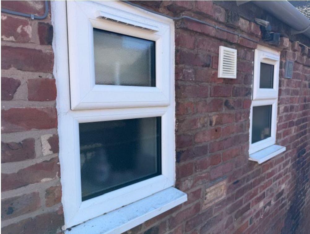
Fig 6. Flat 5A obscured windows
