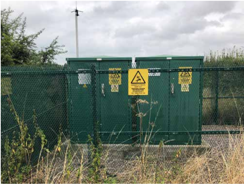
Electrical substation at north-western Site boundary
