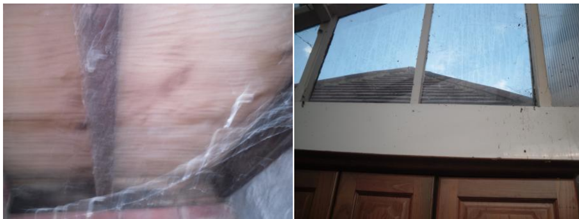
Inside outside toilet (Boarding under felt): cobwebbed and view of garage roof from inside plastic linkway
