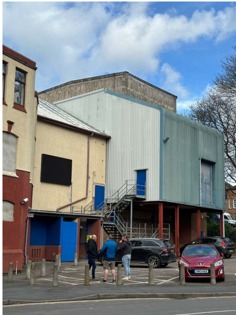
Poor quality finish of stage house will be replaced.
