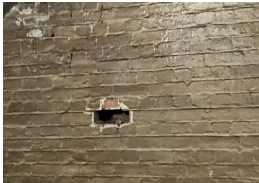
Photograph 5: missing bricks at south gable of internal void of B1
