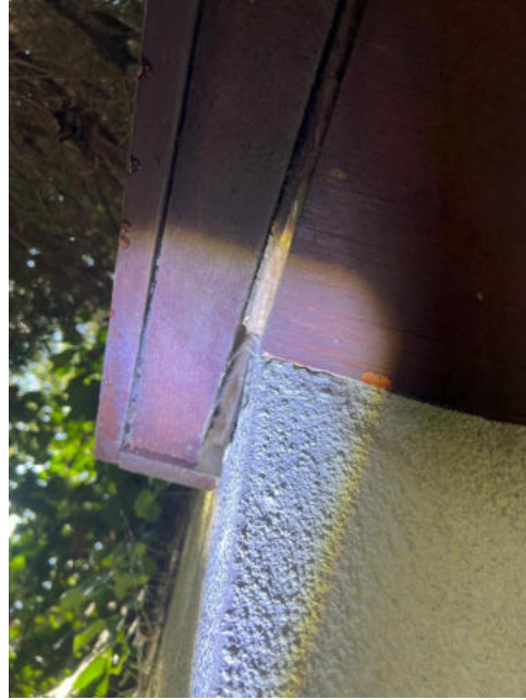
Photo 10: Gaps in building B1 barge boards
