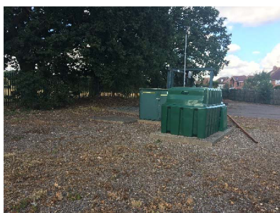
Photo 10: View of Severn Trent Water Sewage Pumping Station north of Field 2
