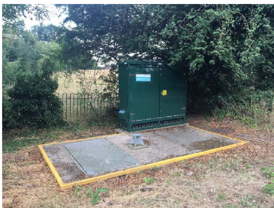
Photo 11: View of Severn Trent Water Sewage Pumping Station north of Field 1
