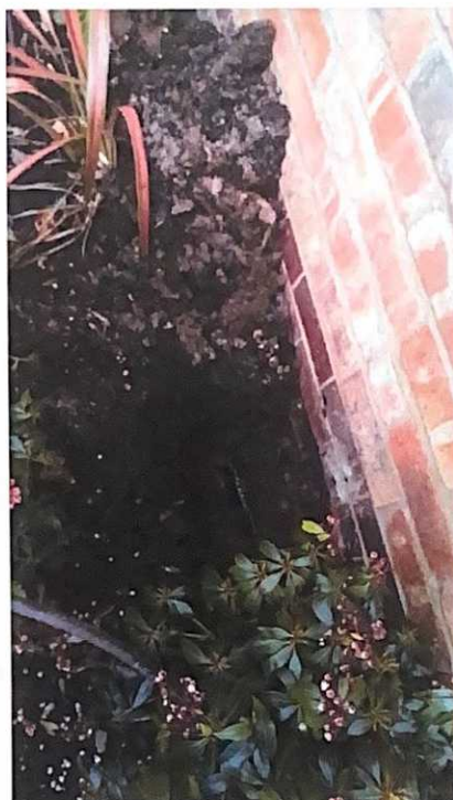
Plate 7: Second small trench advanced in the flower bed showing free phase oil above the footing
