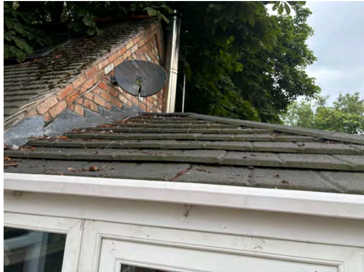
Image 7 - Condition of roof tiles on conservatory.
