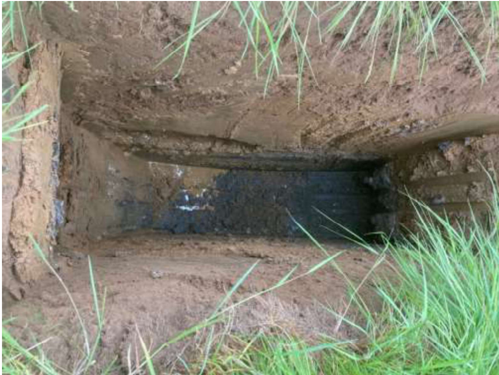
TP34 – Trial Pit
