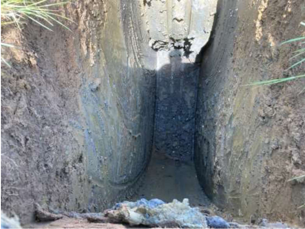
TP41 – Trial Pit
