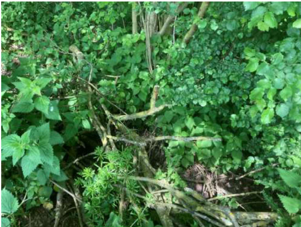
Looking north showing covered ditch blocked with plant debris
