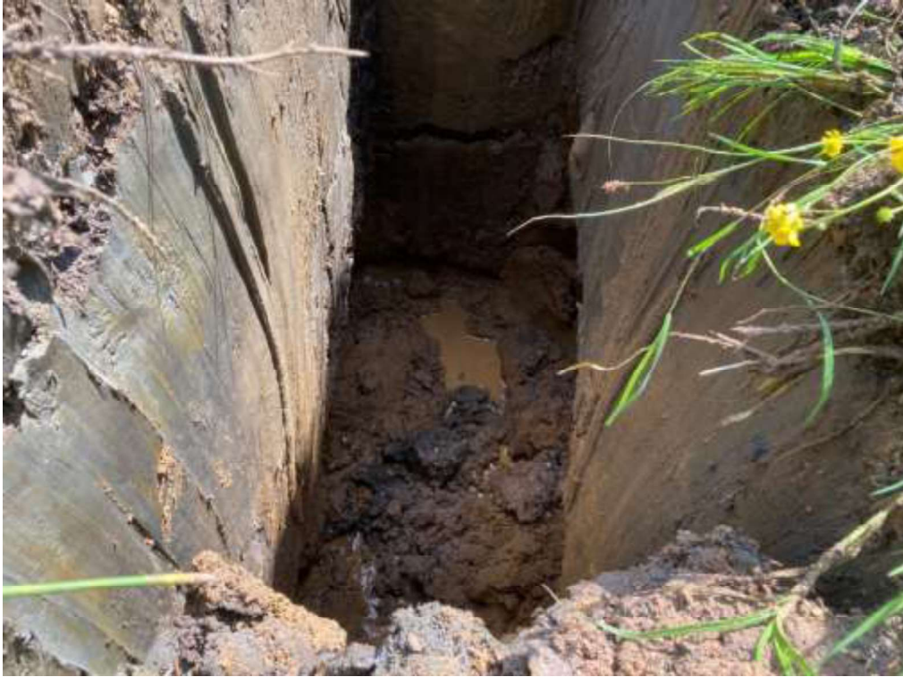
TP06 – Trial Pit
