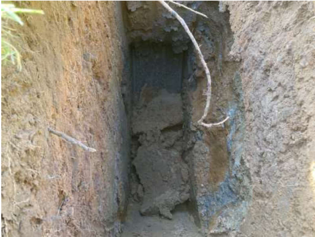
TP01 – Trial Pit
