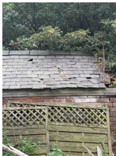
Plate 14. Roof in disrepair
