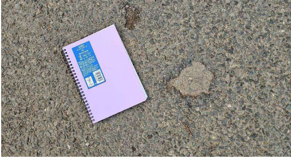
Figure 111: Small Defect in Tarmac 400m East of the Lychgate Lane Junction
