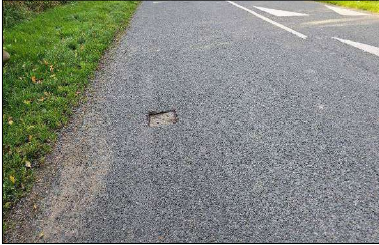
Figure 100: General Carriageway Condition East of Lychgate Lane Junction
