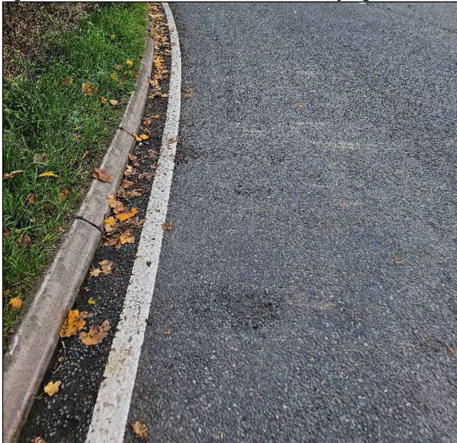
Figure 101: Small Tarmac Defects 1.6km east of Lychgate Lane Junction
