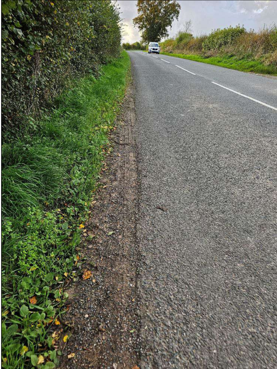
Figure 103: Edge of Carriageway Tarmac Damage 1.4km east of Lychgate Lane Junction
