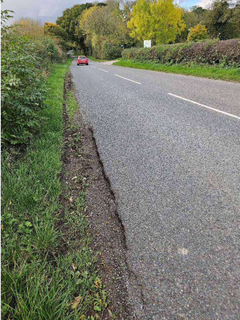
Figure 110: Damage to Edge of Carriageway 450m East of Lychgate Lane Junction
