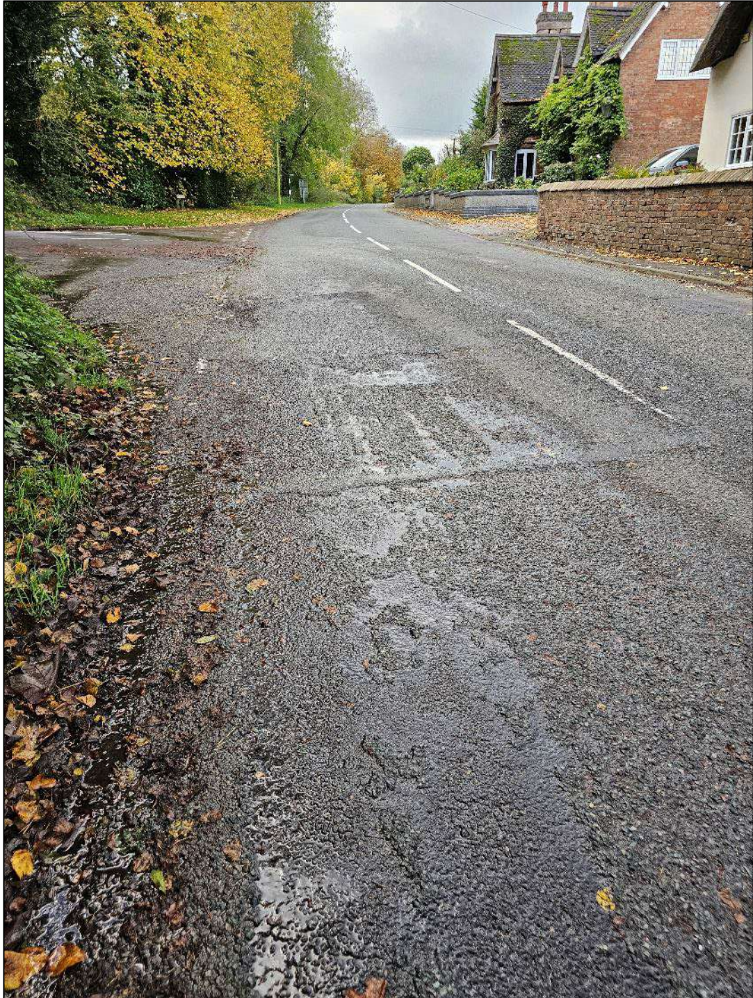
Figure 117: General Carriageway Condition Immediately East of the Lychgate Lane Junction. Defects Visible Within Tarmac.
