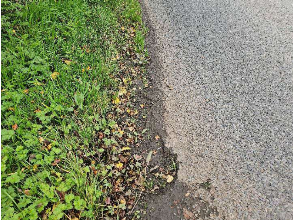
Figure 109: Damage to Edge of Carriageway 700m East of Lychgate Lane Junction
