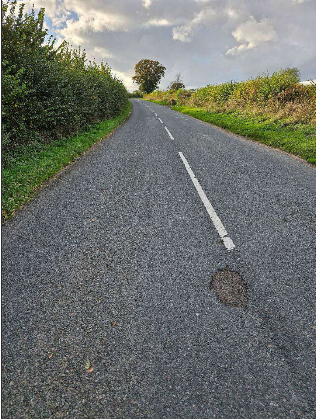
Figure 102: Small Carriageway Defects 1.4km east of Lychgate Lane Junction
