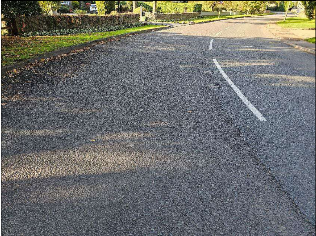
Figure 97: General Carriageway Condition 2.2km east of Lychgate Lane Junction
