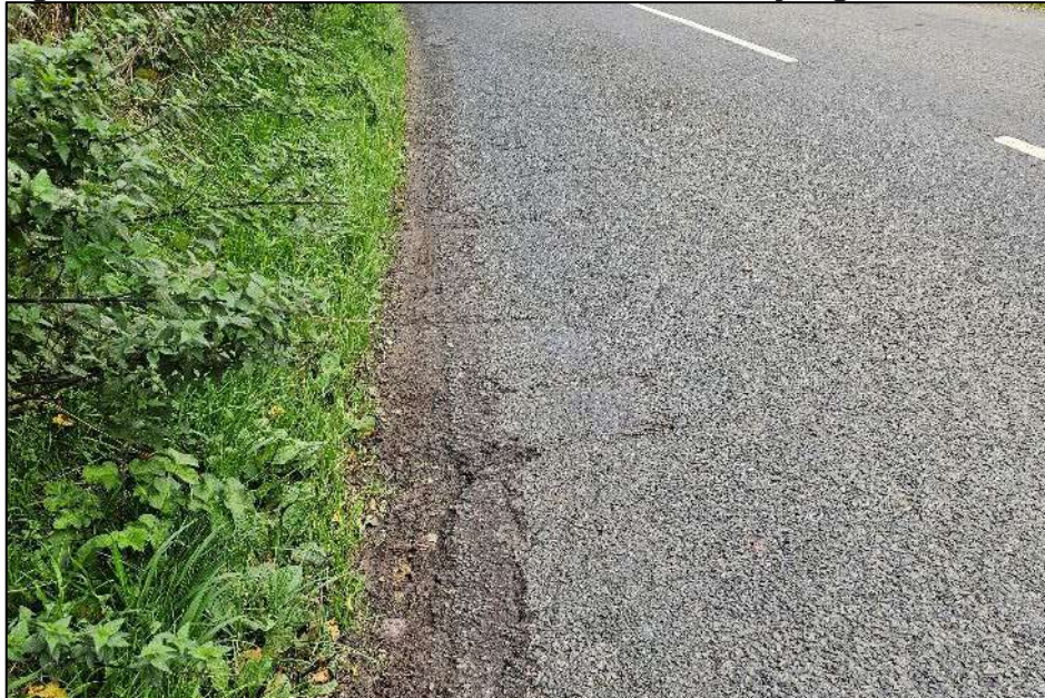
Figure 107: Transverse Cracks 750m East of the Lychgate Lane Junction
