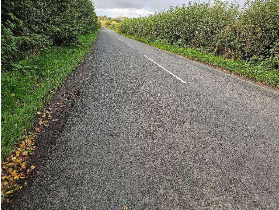
Figure 108: Damage to Edge of Carriageway 725m East of Lychgate Lane Junction
