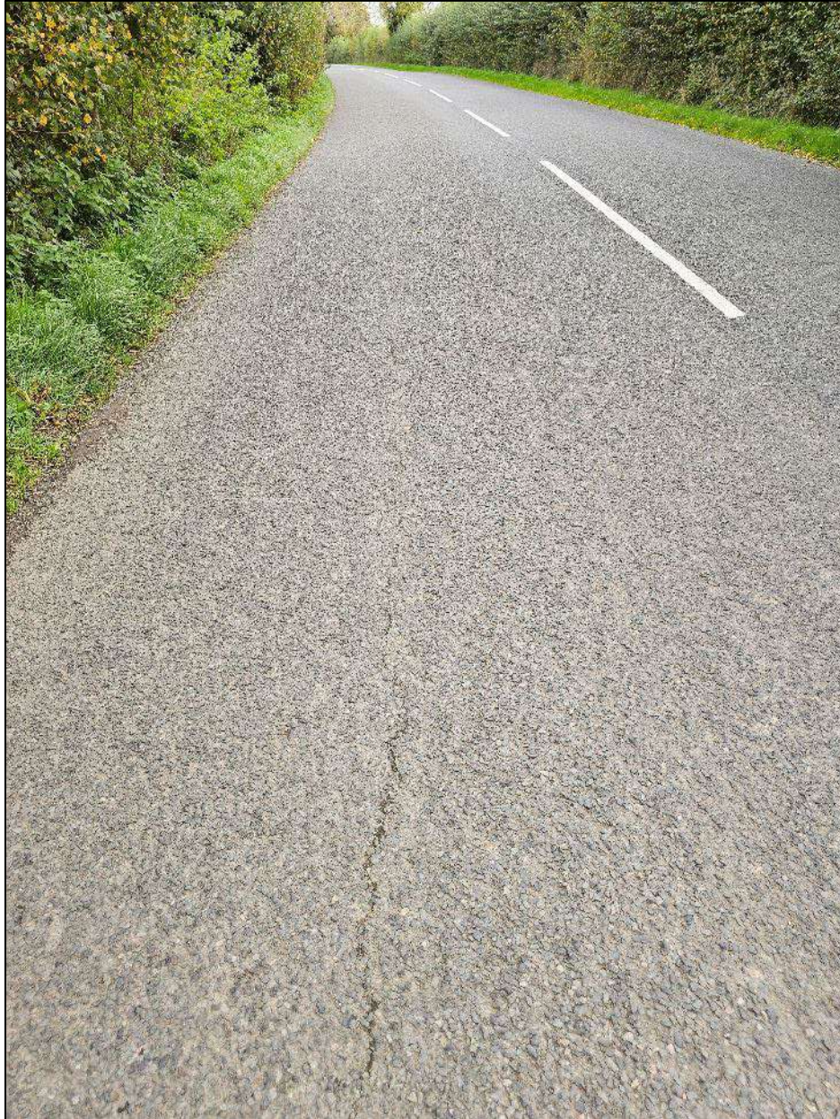
Figure 88: General Carriageway Condition, and Tarmac Surfacing Defect 800m East of Lychgate Lane Junction
