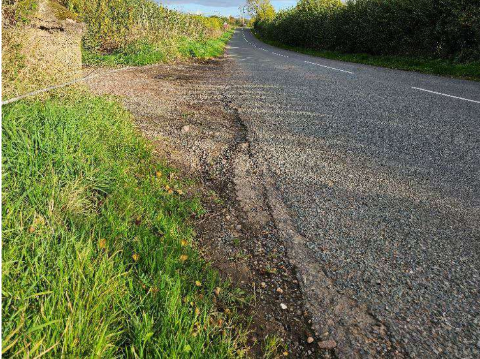
Figure 89: Damage to Edge of Tarmac 1.4km East of Lychgate Lane Junction
