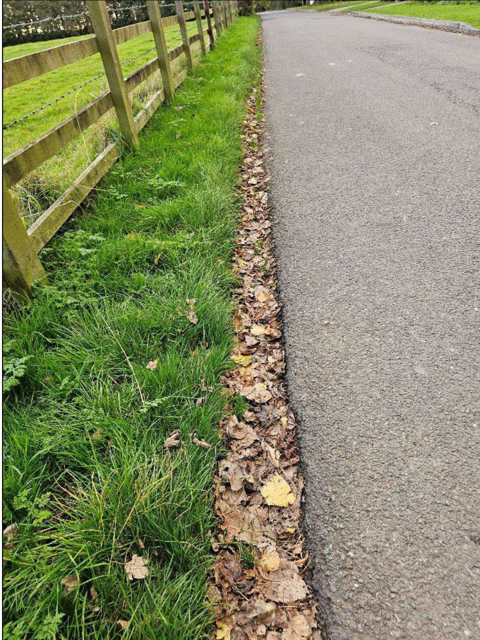
Figure 60: Damage to Grass Verge Approximately 750m East of the Parcel A Access
