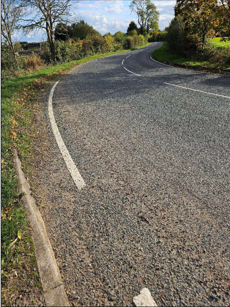
Figure 91: General Carriageway Condition 1.6km East of Lychgate Lane Junction
