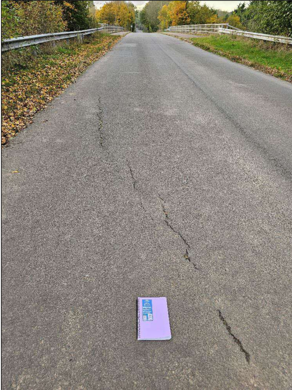
Figure 73: Tarmac Cracks 180m East of the Parcel A Access
