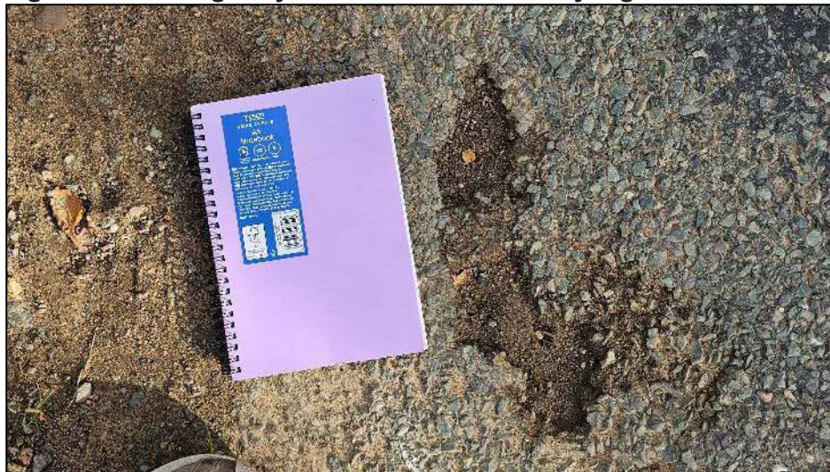
Figure 90: Carriageway Defect 1.4km East of Lychgate Lane Junction
