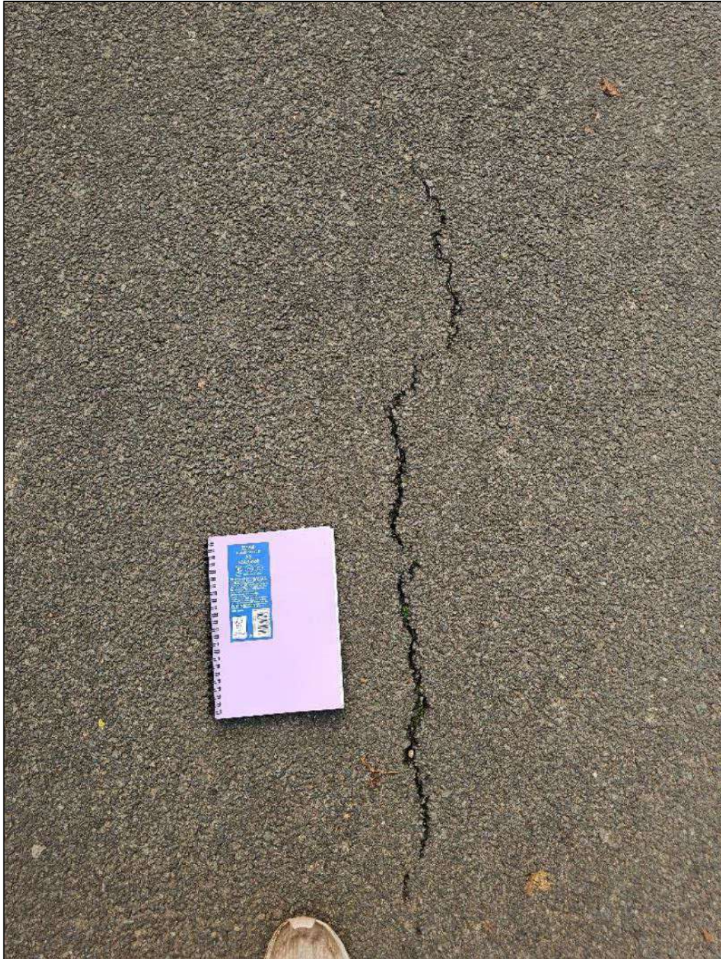
Figure 68: Tarmac Cracks 350m East of the Parcel A Access
