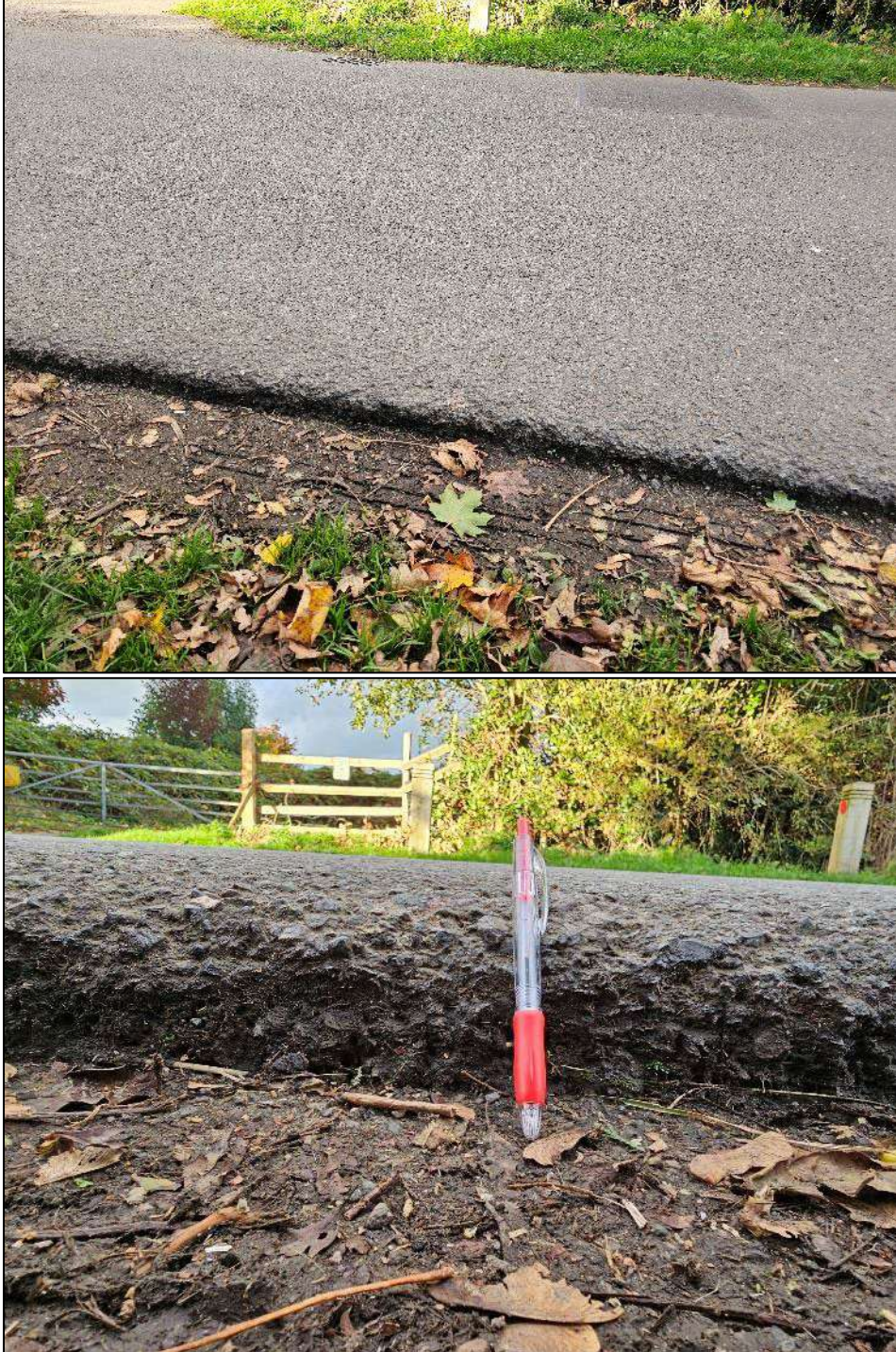
Figure 63: Grass Verge Damage Approximately 700m East of the Parcel A Access
