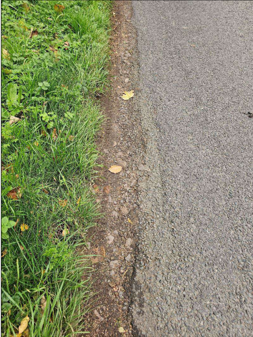
Figure 82: Damage to Surface Level tarmac 100m East of the Lychgate Lane Junction
