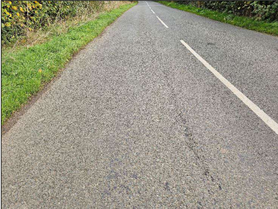
Figure 86: General Carriageway Condition 500m East of Lychgate Lane Junction
