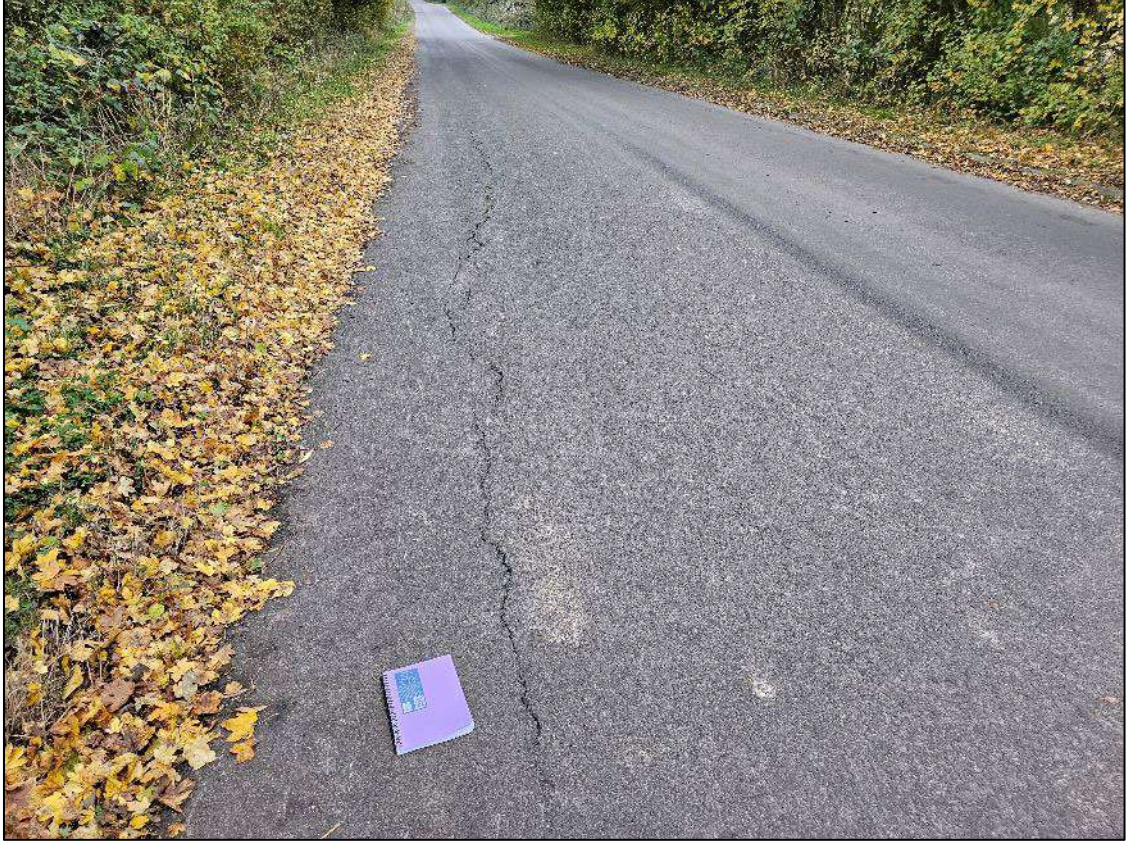
Figure 78: Tarmac Surface Cracks Parallel to Kerblines, 100m East of the Parcel A Access
