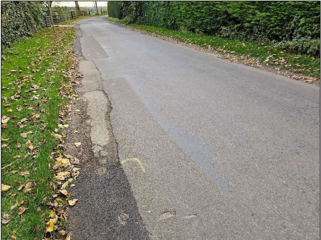
Figure 58: Damage to Edge of Carriageway Approximately 85m East of the Parcel A Access
