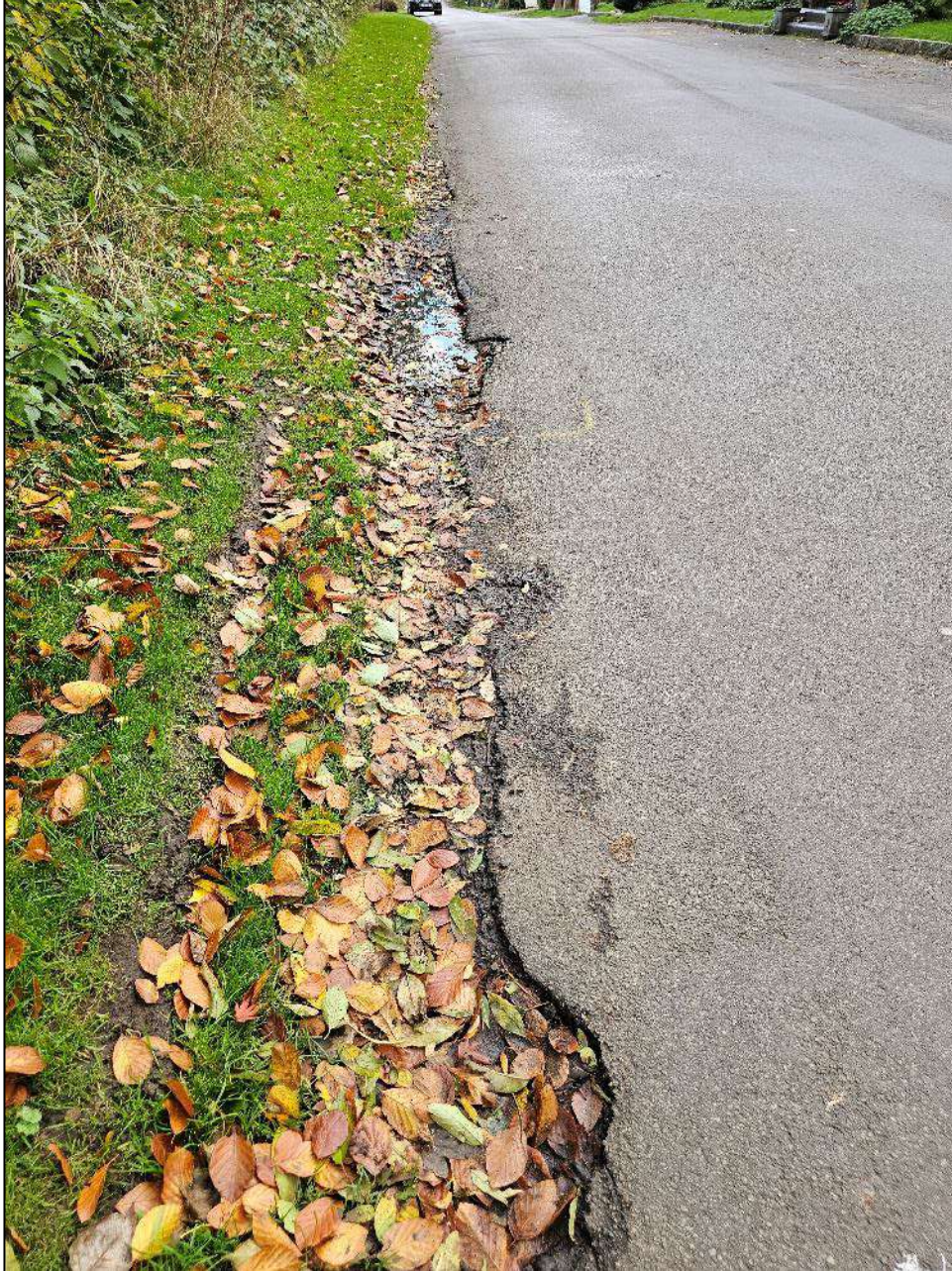
Figure 55: Damage to Edge of Carriageway Approximately 950m East of the Parcel A Access
