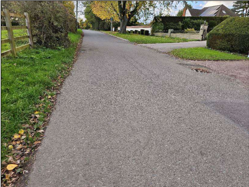
Figure 62: Tarmac Crack Approximately 750m East of the Parcel A Access
