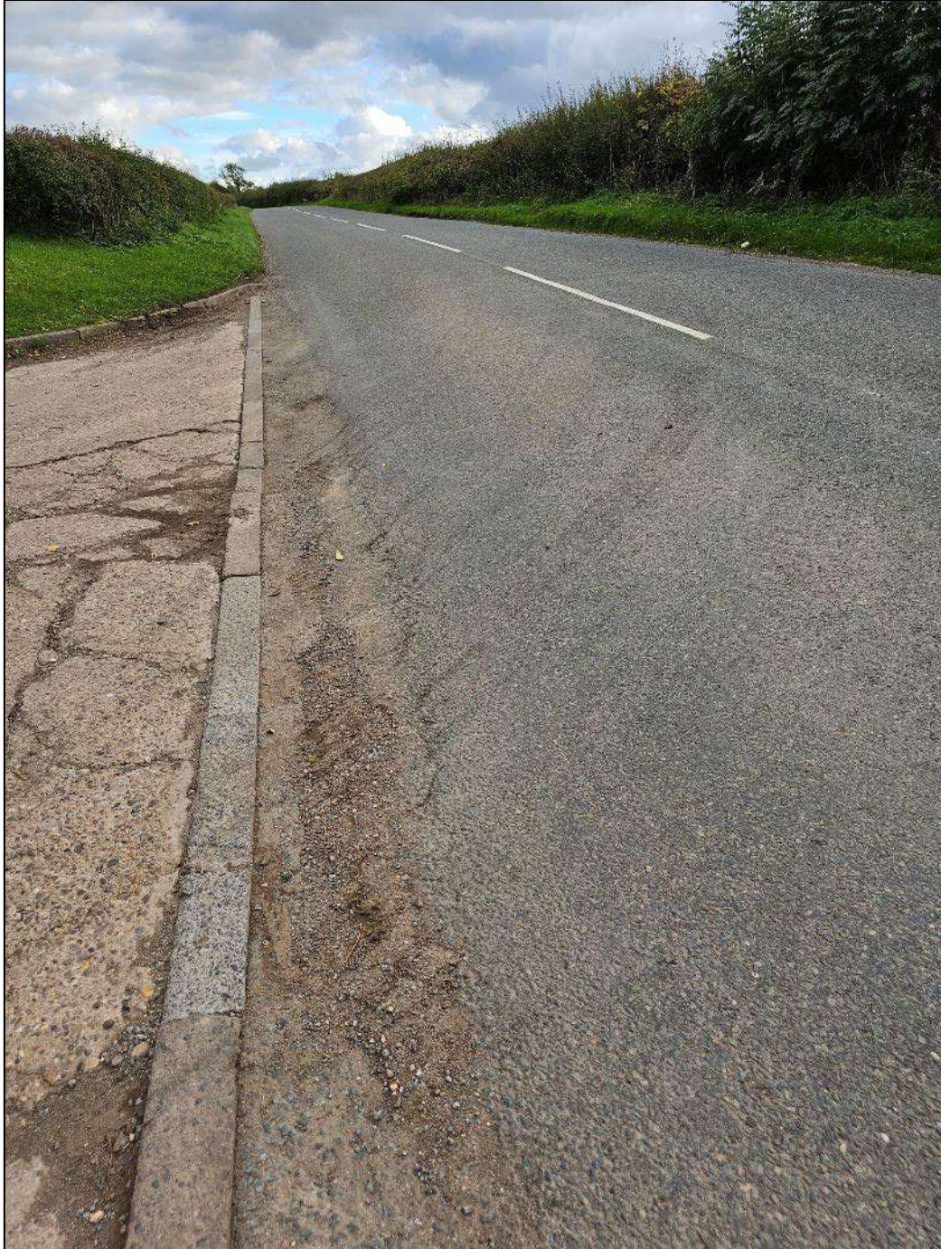
Figure 84: General Carriageway Condition at Green Waste Recycling Access, 400m East of Lychgate Lane Junction
