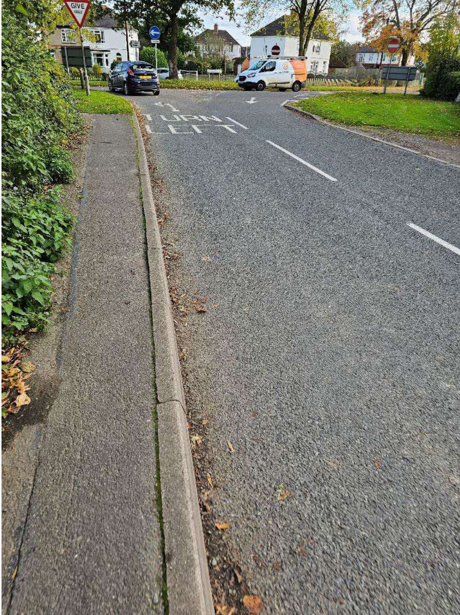
Figure 96: General Tarmac Condition 2.1km East of Lychgate Lane Junction
