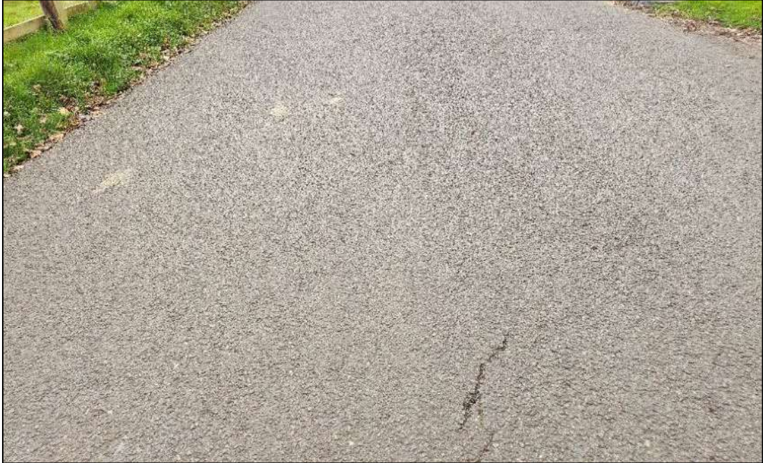
Figure 61: Tarmac Crack Approximately 750m East of the Parcel A Access
