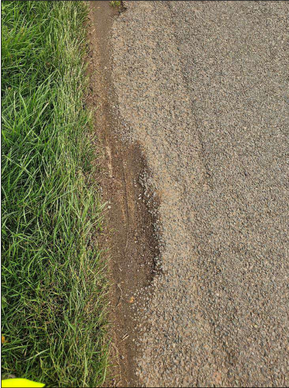
Figure 85: Damage to Edge of Tarmac 450m East of Lychgate Lane Junction
