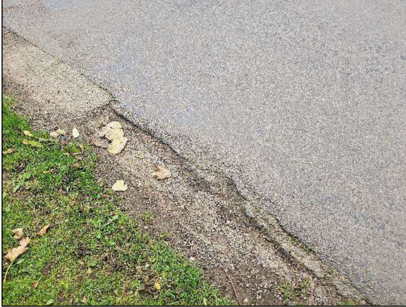
Figure 57: Damage to Edge of Carriageway Approximately 85m East of the Parcel A Access
