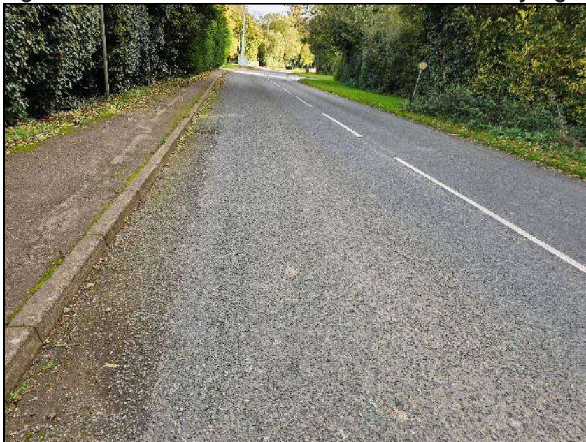
Figure 94: General Tarmac Condition 1.8km East of Lychgate Lane Junction
