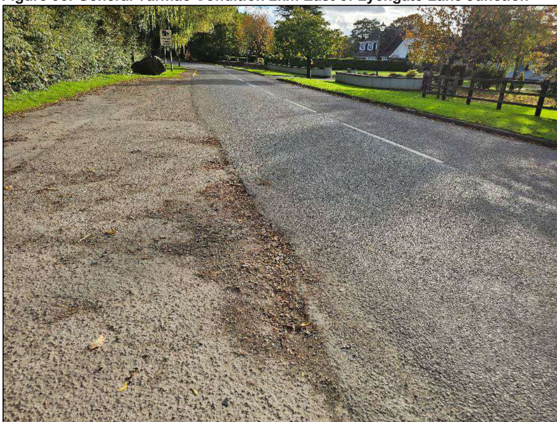
Figure 95: General Tarmac Condition 2km East of Lychgate Lane Junction
