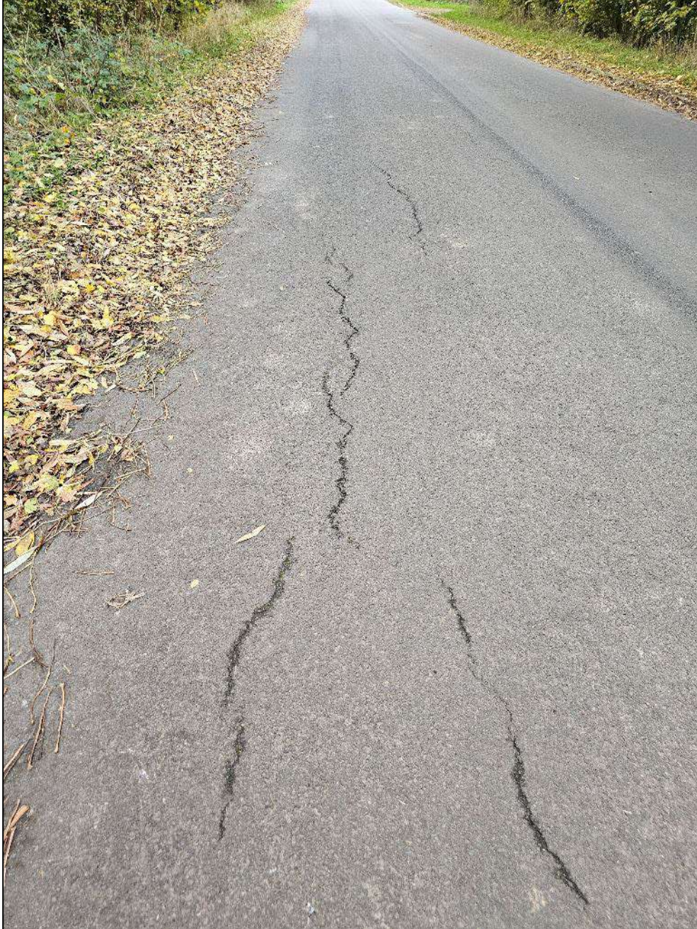
Figure 79: Tarmac Surface Cracks Parallel to Kerblines, 65m East of the Parcel A Access
