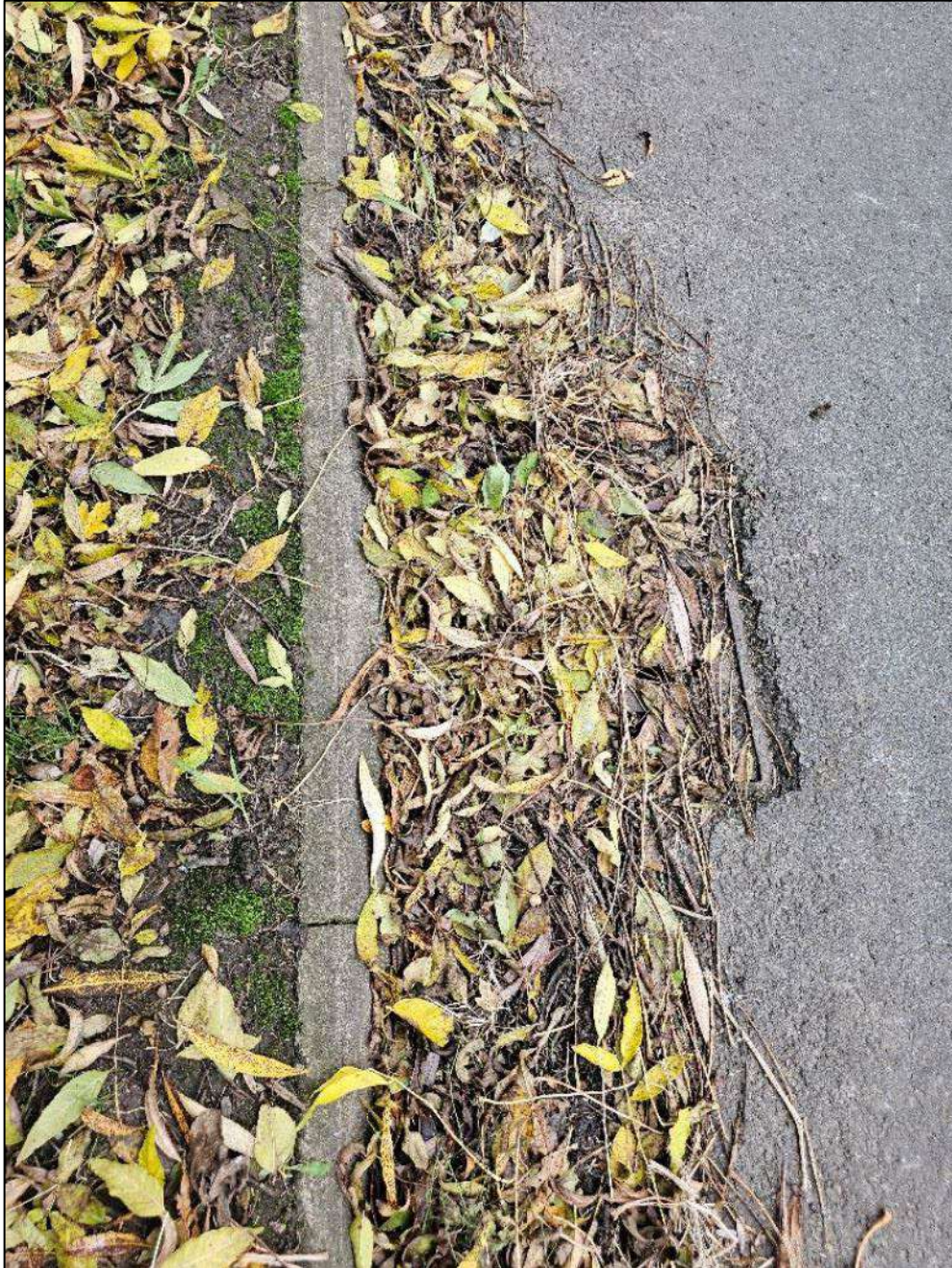
Figure 8: Drain Obstructed by Debris 40m East of the Parcel A Access
