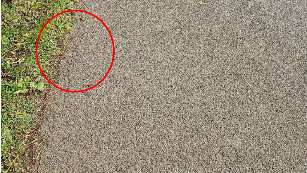
Figure 35: Shallow Tarmac Defect Approximately 700m East of the Parcel A Access
