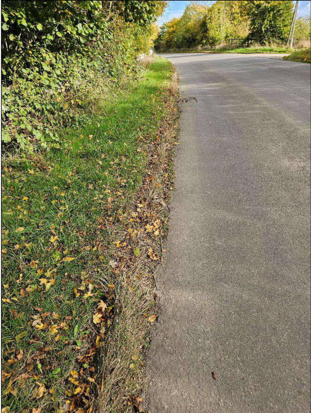
Figure 23: Kerblines and Tarmac Condition 225-230m East of the Parcel A Access
