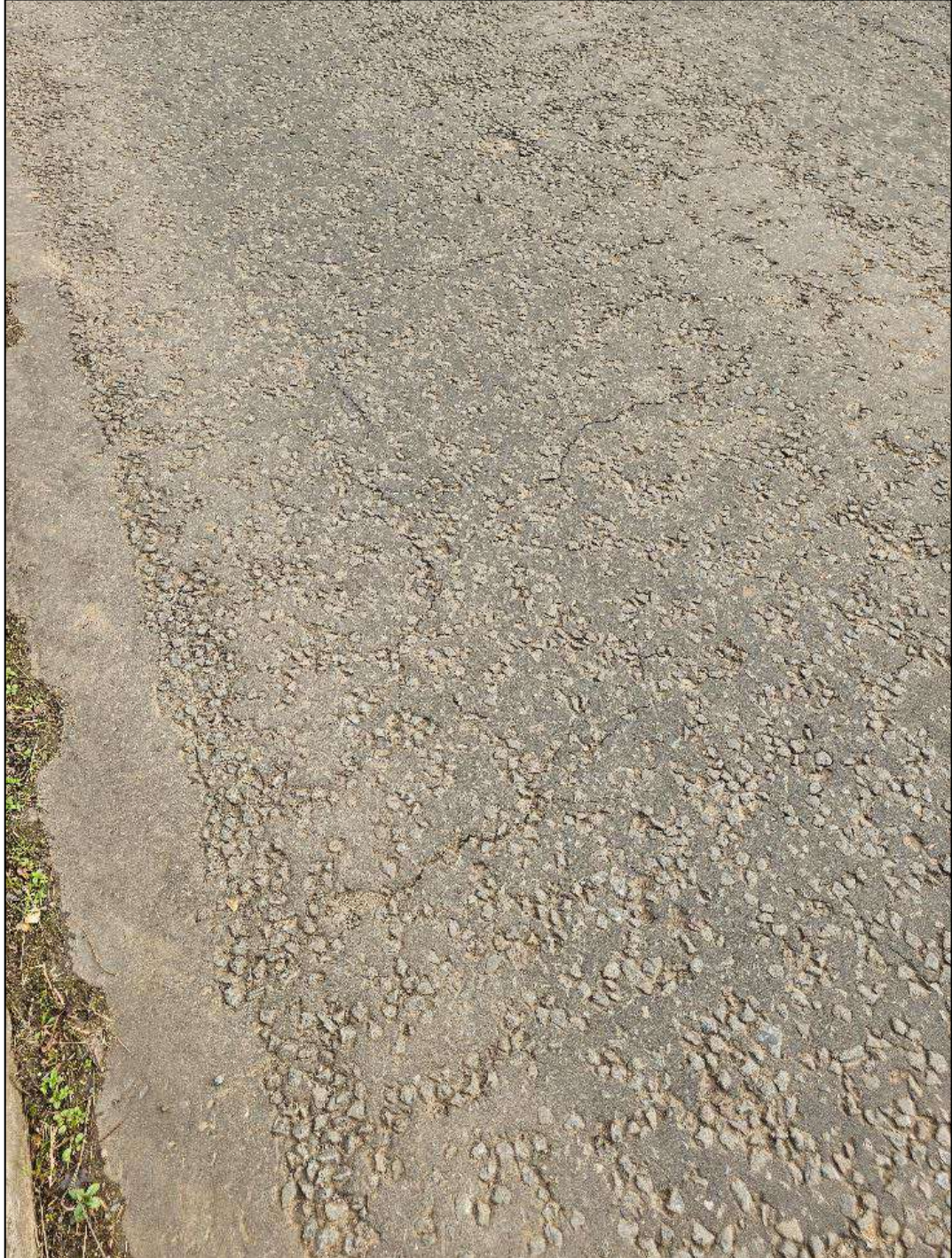
Figure 17: Surface Tarmac Shallow Cracks 130m East of the Parcel A Access
