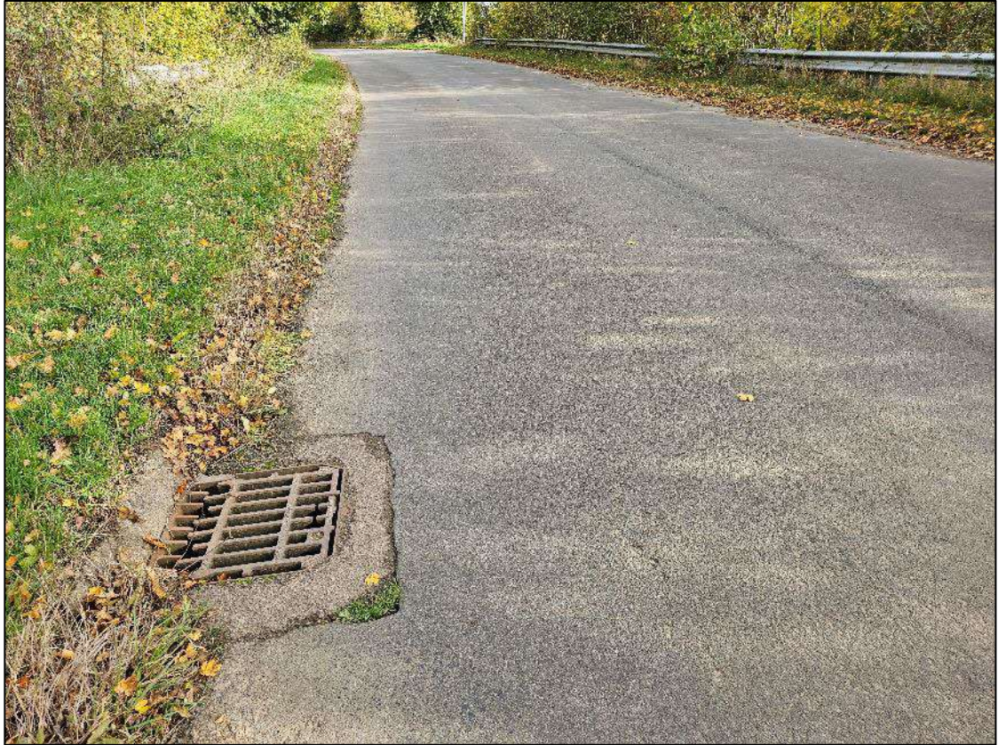
Figure 20: Drain and Carriageway Condition 220m East of the Parcel A Access
