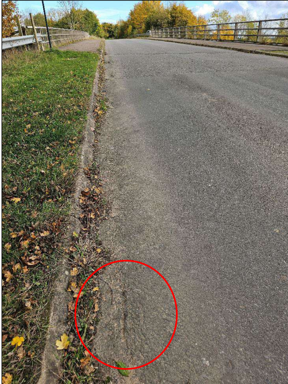
Figure 12: Defect in Carriageway 115m east of the Parcel A Access
