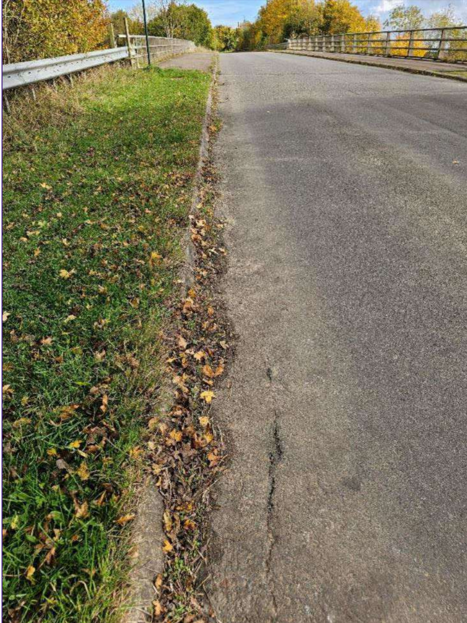
Figure 10: Defect in Carriageway 110m east of the Parcel A Access
