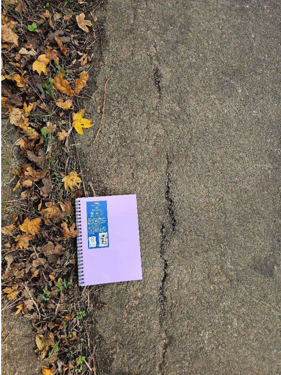
Figure 11: Defect in Carriageway 110m east of the Parcel A Access
