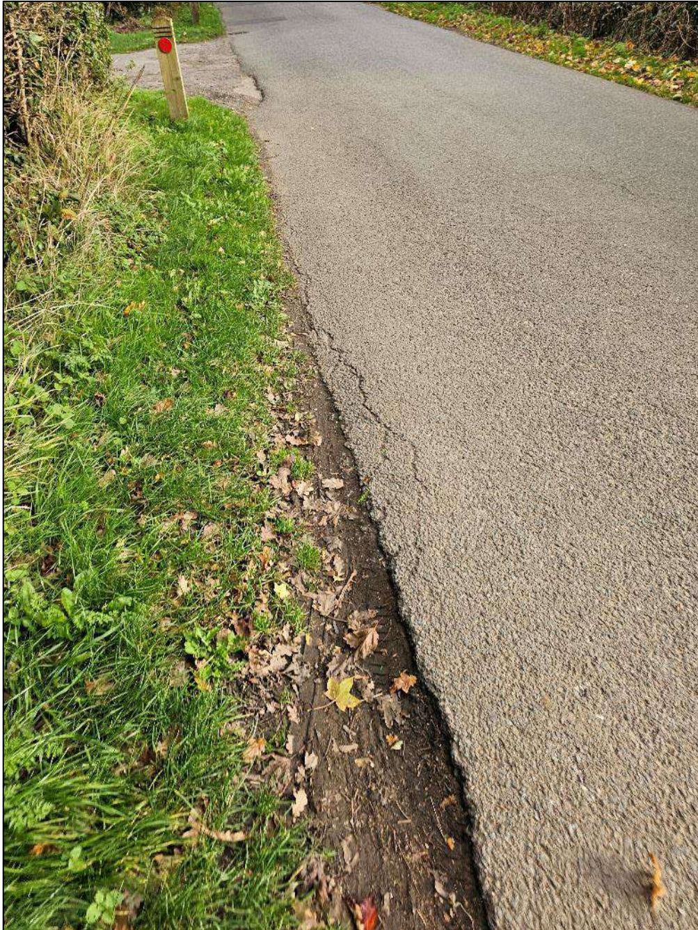
Figure 34: Grass Verge Degradation and Tarmac Defect 670-680m East of the Parcel A Access
