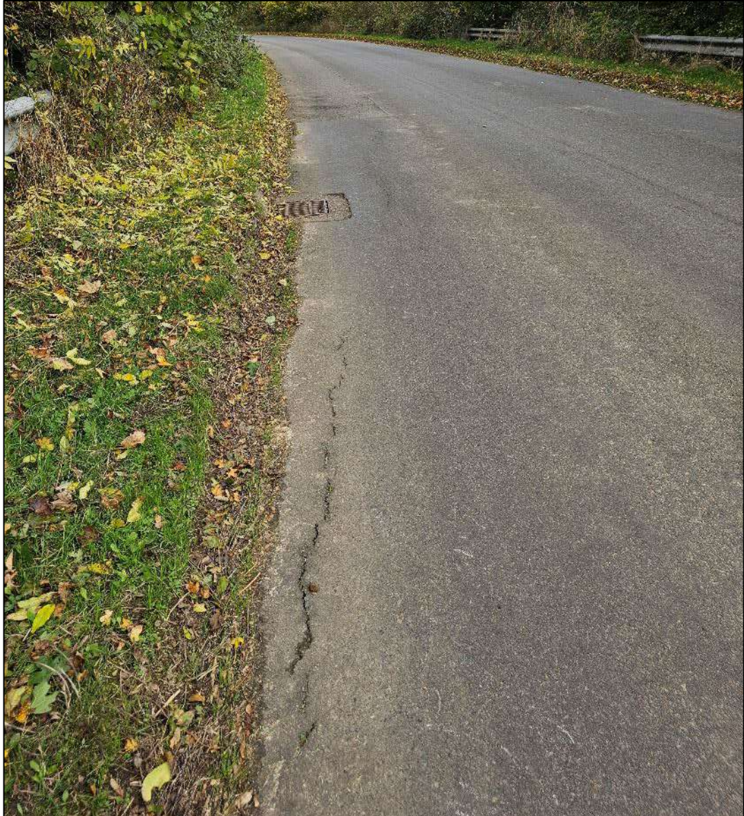
Figure 27: Kerbline and Tarmac Condition 280m East of the Parcel A Access. Surface Defects Run Parallel to Kerbline
