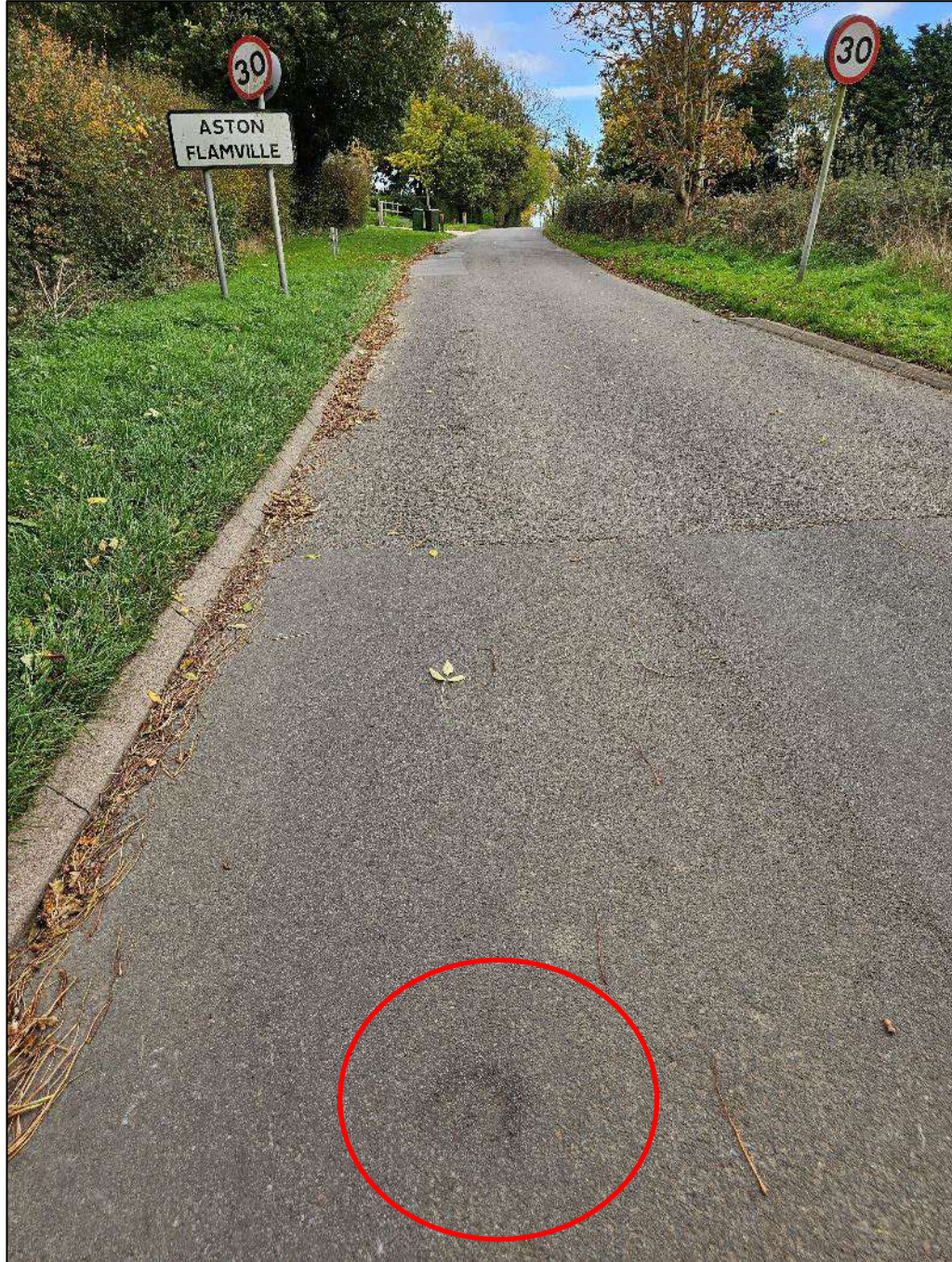
Figure 30: Kerbline and Tarmac Condition Approximately 520m East of the Parcel A Access.
