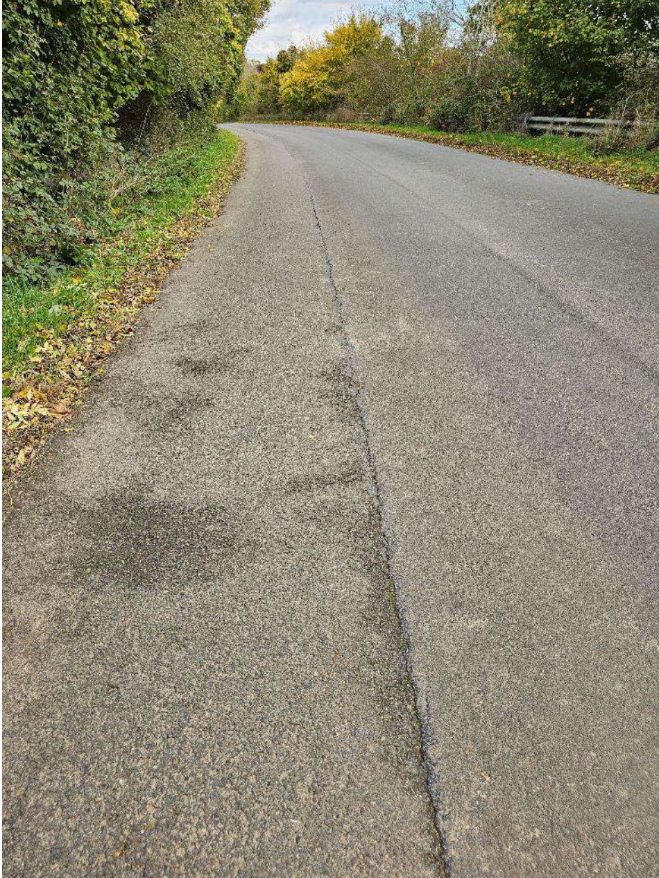
Figure 28: Kerbline and Tarmac Condition 280-290m East of the Parcel A Access. Surface Defects Run Parallel to Kerbline
