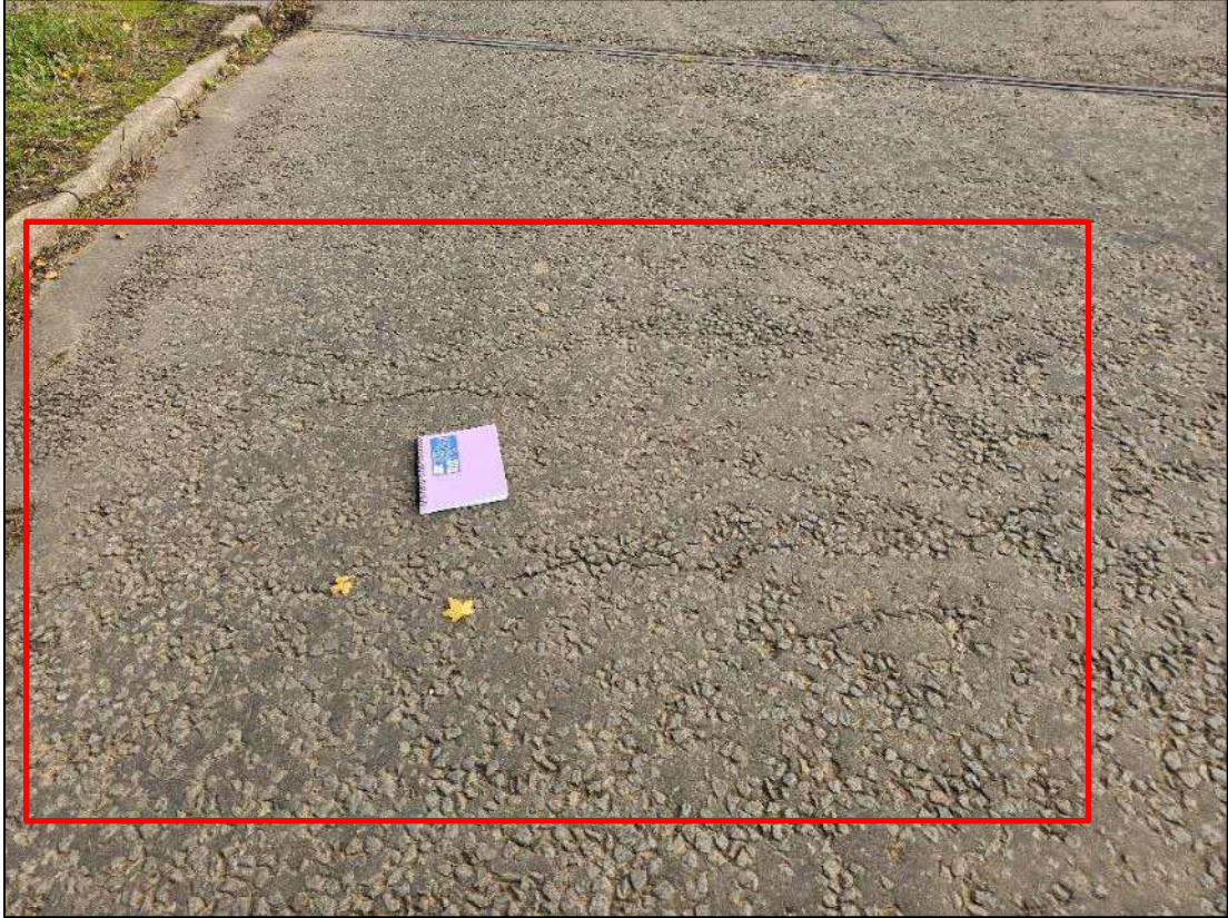
Figure 15: Shallow Transverse Cracks 125m East of the Parcel A Access
