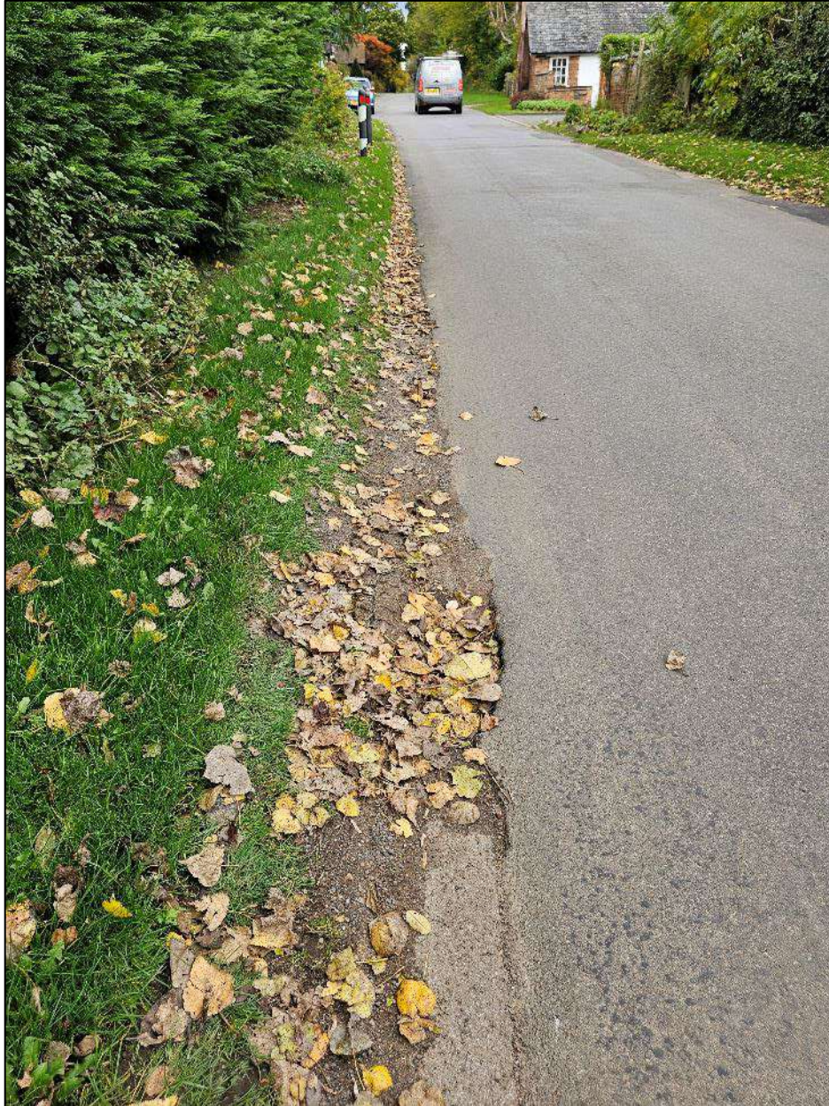
Figure 38: Defects on Edge of Carriageway Approximately 900m East of the Parcel A Access
