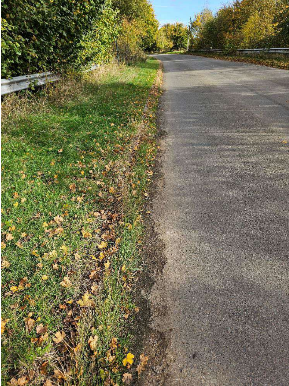
Figure 19: Kerblines and Tarmac Condition 200m East of the Parcel A Access
