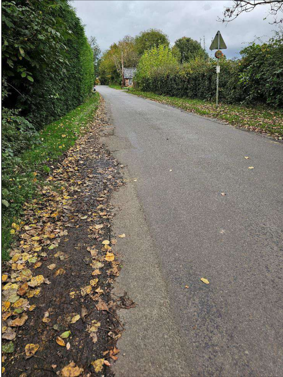
Figure 37: General Carriageway Condition Approximately 850m East of the Parcel A Access
