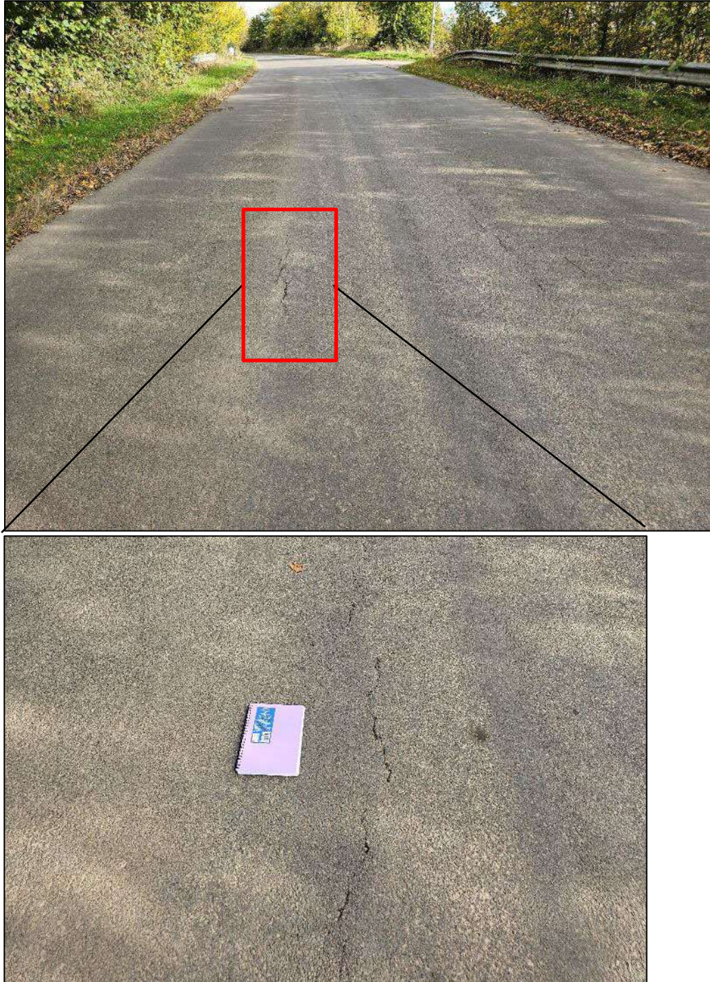
Figure 21: Tarmac Cracks 220m East of the Parcel A Access
