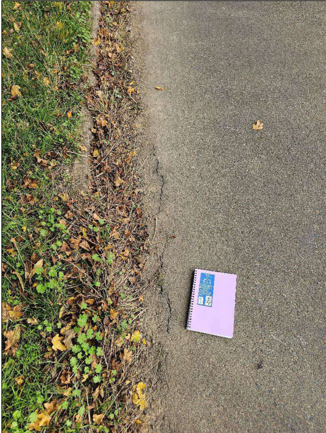
Figure 18: Cracks in Tarmac Running Parallel to Kerbing, 210m East of the Parcel A Access
