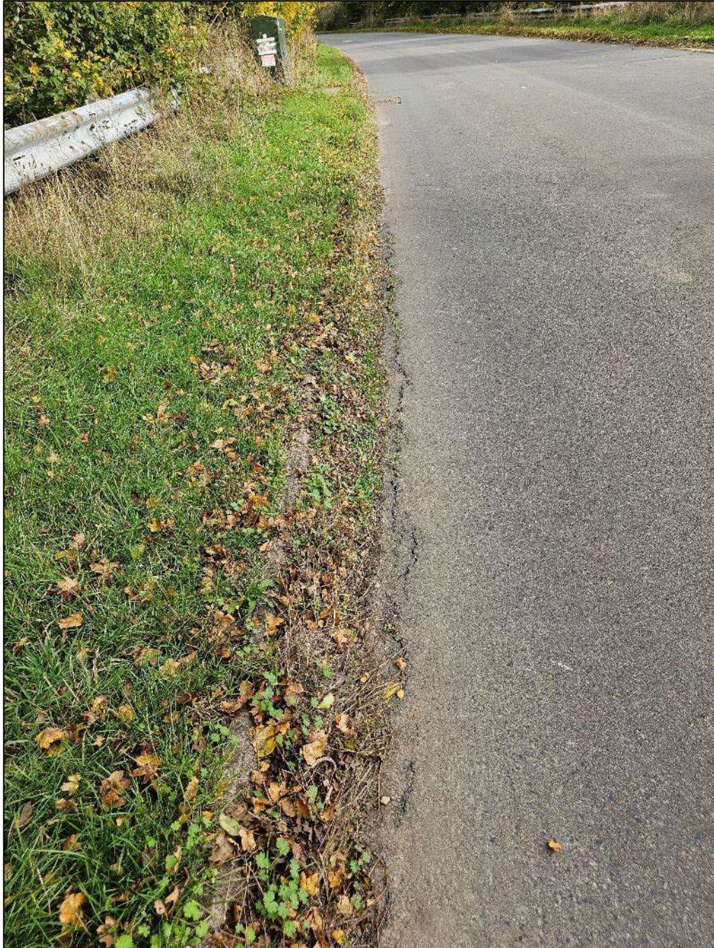
Figure 24: Kerbline and Tarmac Condition 250m East of the Parcel A Access. Surface Defects Run Parallel to Kerbline
