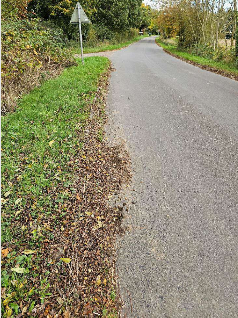
Figure 29: Kerbline and Tarmac Condition 450m East of the Parcel A Access. Debris Adjacent to Kerbline
