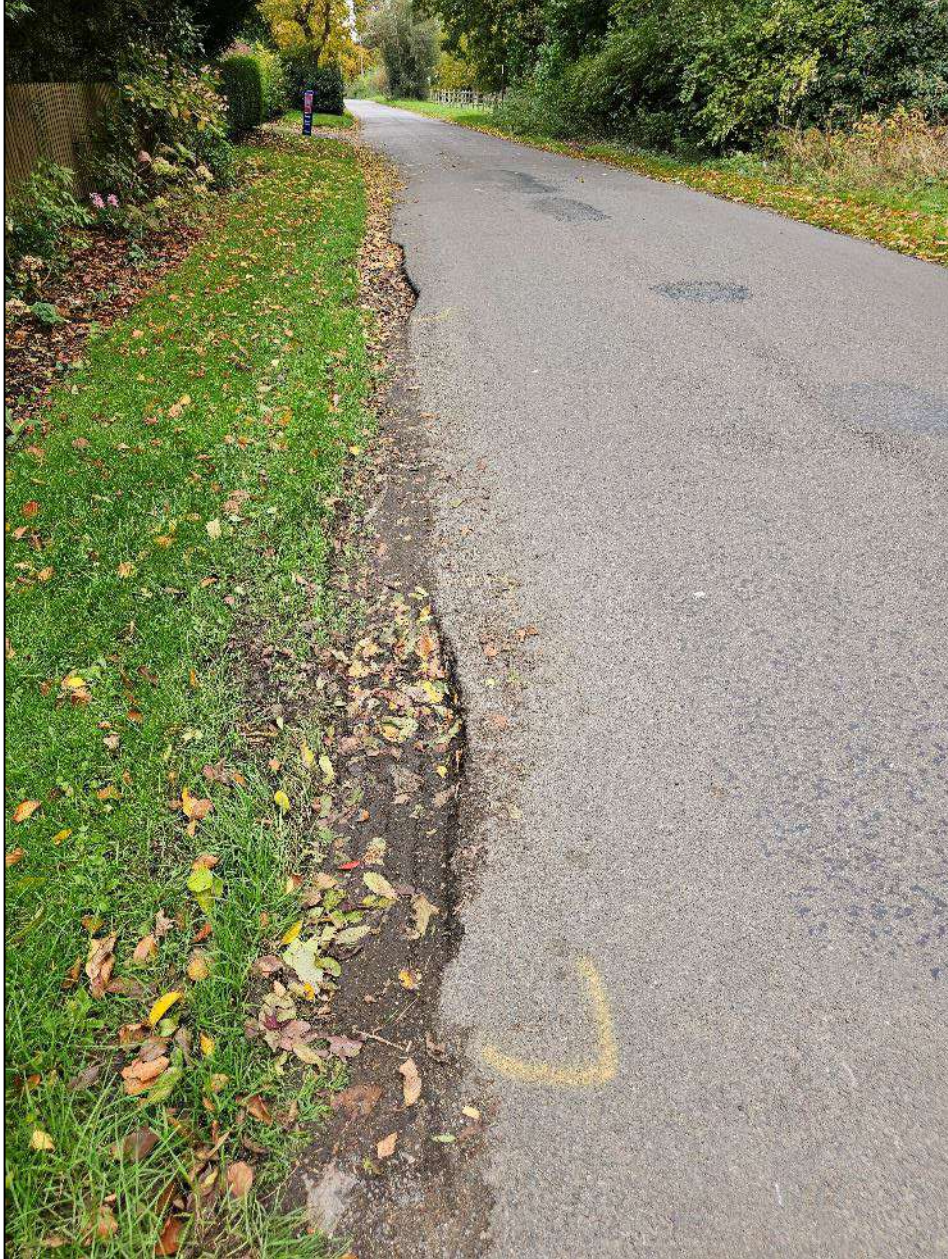
Figure 43: Breakup of Tarmac Surfacing at Edge of Carriageway Approximately 1000m East of the Parcel A Access
