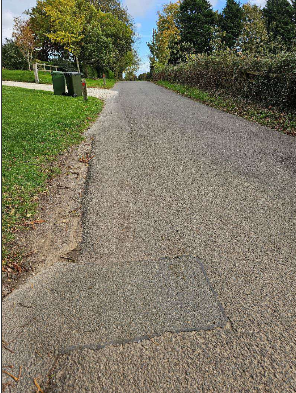
Figure 31: Carriageway Patching and General Carriageway Condition Approximately 600m East of the Parcel A Access.
