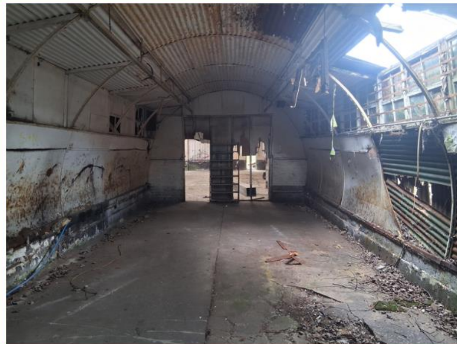
Photo No.18: Dilapidated former Nissen-hut adjoined to onsite structures
