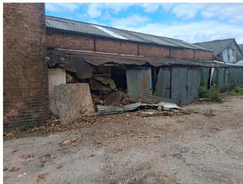
Photo No.28: Facing north showing the southern face of the dilapidated, centrally located workshop structures
