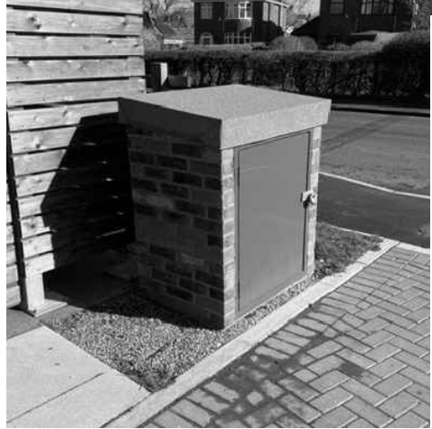
Landlords Feeder Pillar Enclosure
