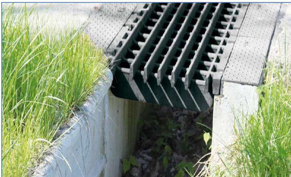
Example of GCN tunnel under a road
