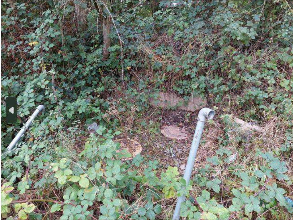
Photograph 7: Existing petrol interceptor in north east corner of site
