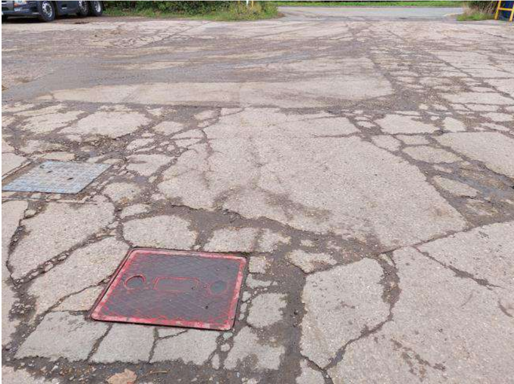
Photograph 5: Colour-coded drains and cracked hardstanding at site entrance
